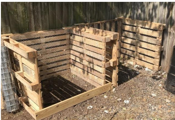
Double 2.4 m wide (two standard pallets) x 1.0 m depth (one standard pallet)
